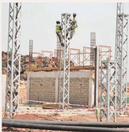
GREEN ENERGY The Turkana Wind Power substation project in Laisamis in Marsabit. The wind farm is touted as Africa's largest. --FILE
